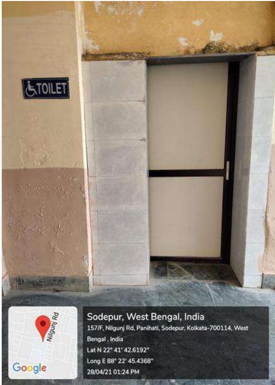
Toilet for Disabled Staffs
