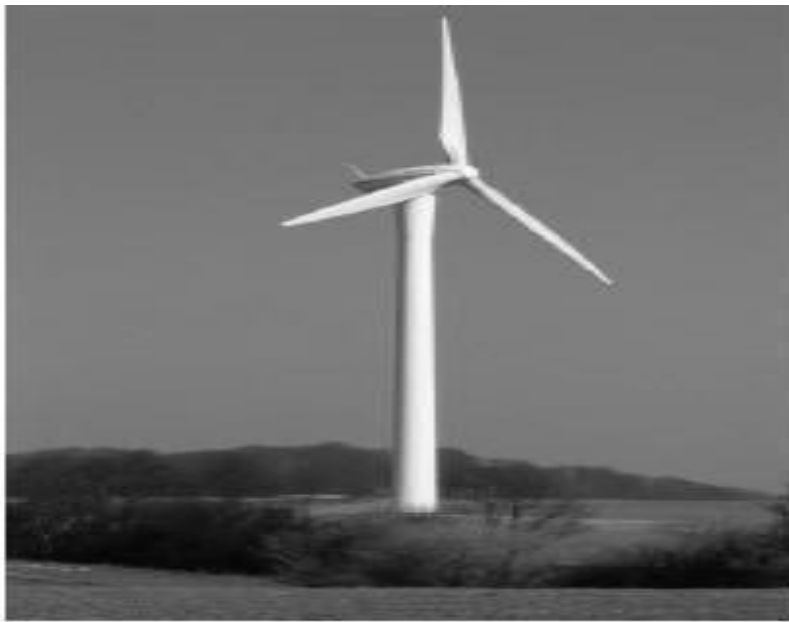
Wind Turbine Generator units
